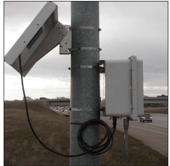
Bluetooth Detector with Cellular Communications and Solar Power
